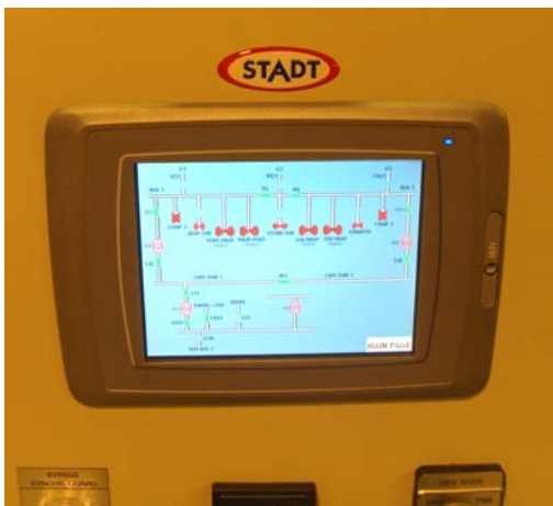
POWER MANAGEMENT SYSTEM
