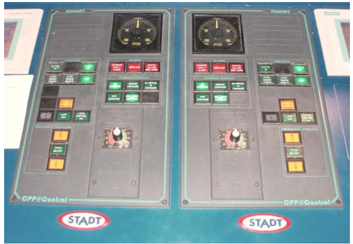
CONTROL ROOM PANELS STASCHO
